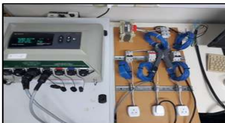
Fig. 4. Square-D PCM4000 network analyzer and test board
