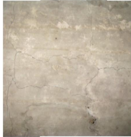
Figure 6. Original crack in concrete
