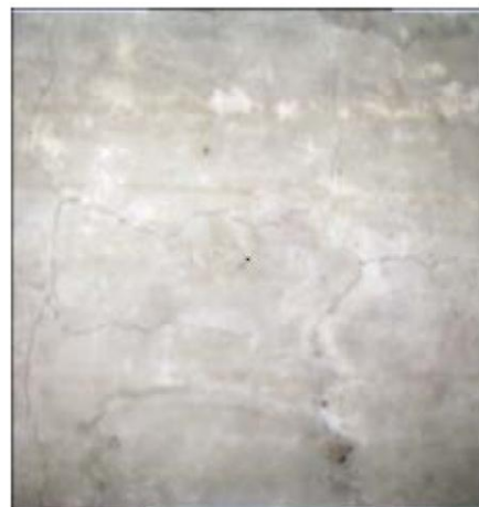
Figure 8. Reconstructed crack in concrete
