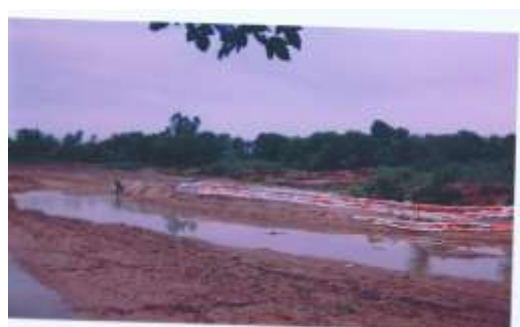
Plate 3: Row of sand bags across the main flow to control the shift of channel, a practice adopted by local people
