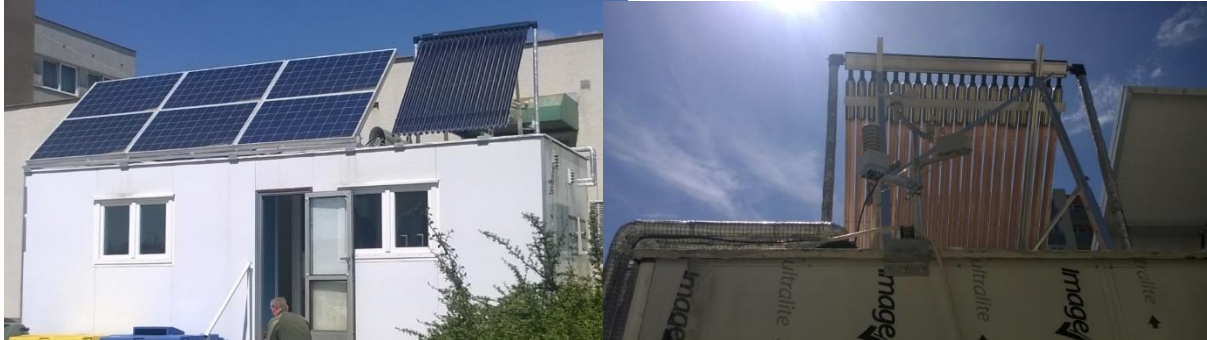
FIG. 3 Mobile laboratory - photovoltaic and solar thermal panels, meteorological station [Photo source: authors]
