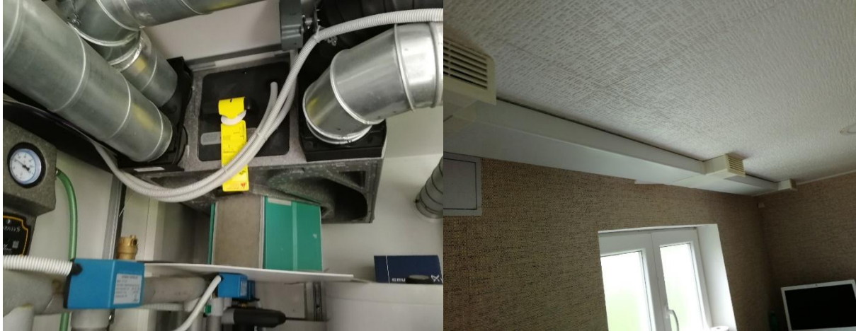
FIG. 8 View of the recuperation ventilation unit and air ductwork in the measuring room [Photo source: authors]
