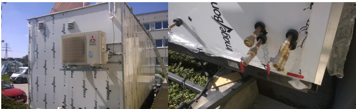
FIG. 5 View of the heat source - heat pump and the possibility of connecting a mobile laboratory to an external heat source [Photo source: authors]
